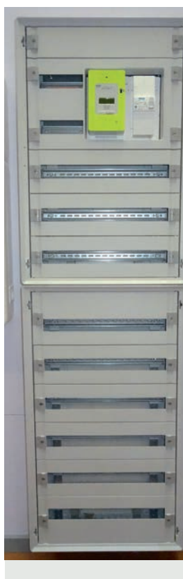
Set of 2 joined cabinets, with meter and incoming circuit breaker at the supply end
