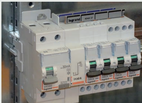
It is possible to mix circuit breakers with automatic and screw terminals on the same row
