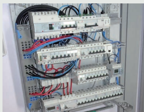
Complete cabinet equipped with different distribution systems
