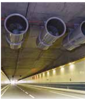
Smoke extractor in a tunnel
