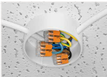
Lighting distribution in ceiling canopy
