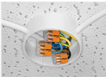
Lighting distribution in ceiling canopy
